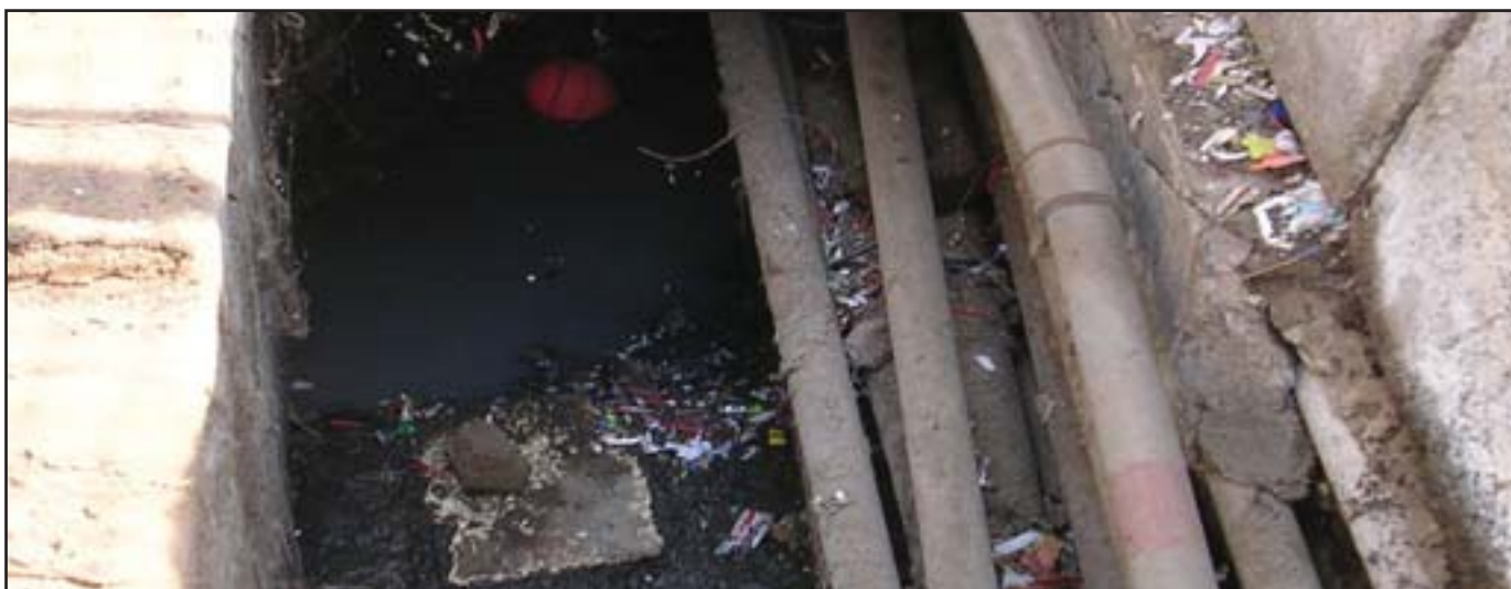
Figure 7: UNHEALTHY WATER... Water pipes running through open sewers and storm water drains are commonplace in Mumbai. [Source: BMC January 2010]
