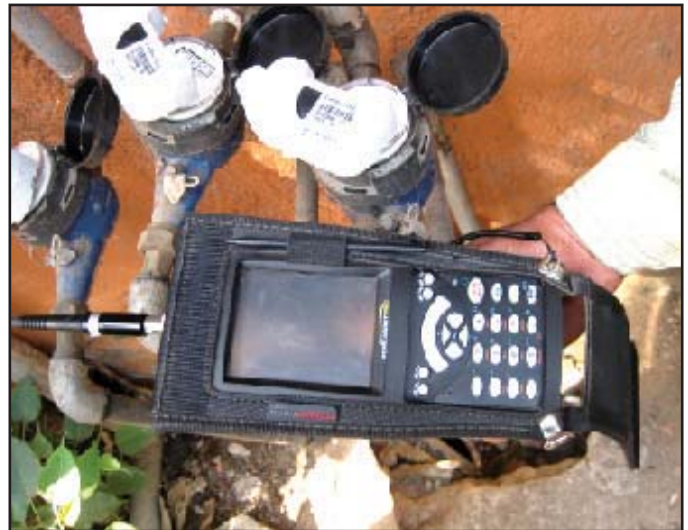
Figure 15: Remotely Aware... GIS-based remote-controlled water meters installed by NMMC. [Source: NMMC]
