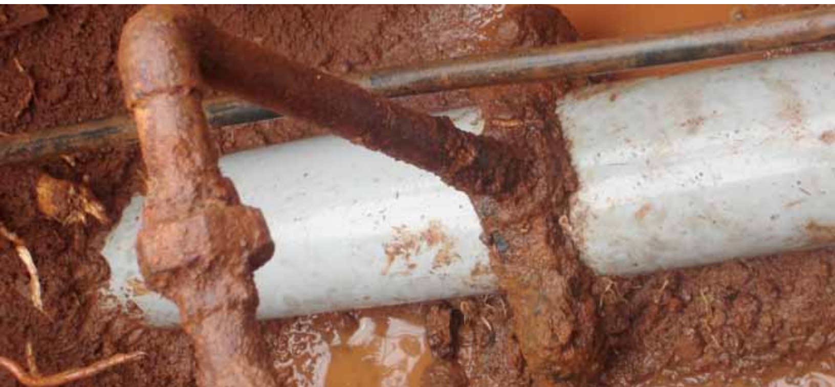
Typical house service connection over unplasticized polyvinyl chloride pipe (conventional method before 24/7 water supply).
