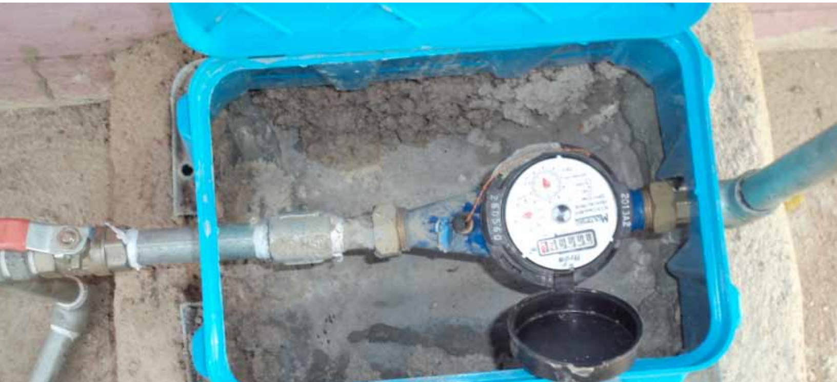
House service connection with customer water meter and protection box.
