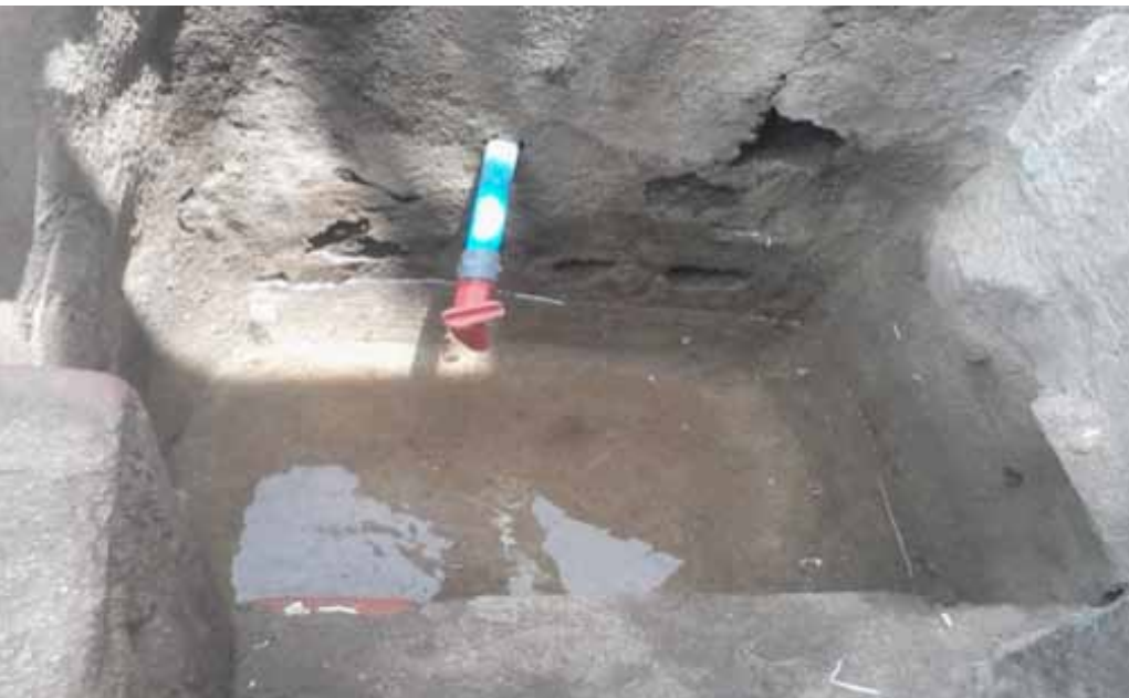
Due to low-pressure and intermittent water supply, many households used a pit or sump in front of their houses to collect water from the substandard services, and the water pumped to a rooftop tank in storing.
