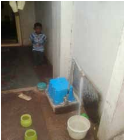
Now with 24/7 water supply, each household has an individual house service connection, receiving water with adequate pressure whenever needed, obviating pit or sump, rooftop tank, and internal pumping.
