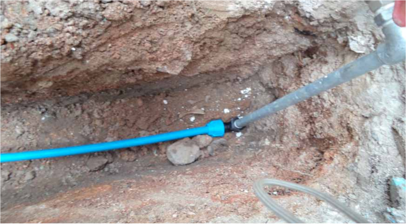
Connecting medium-density polyethylene pipe to galvanized iron pipe for house service connection.
