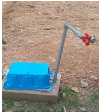
With volumetric tariff, a house service connection with lock system allows customers to lock their taps to prevent water theft and use quality piped water as and when required.
