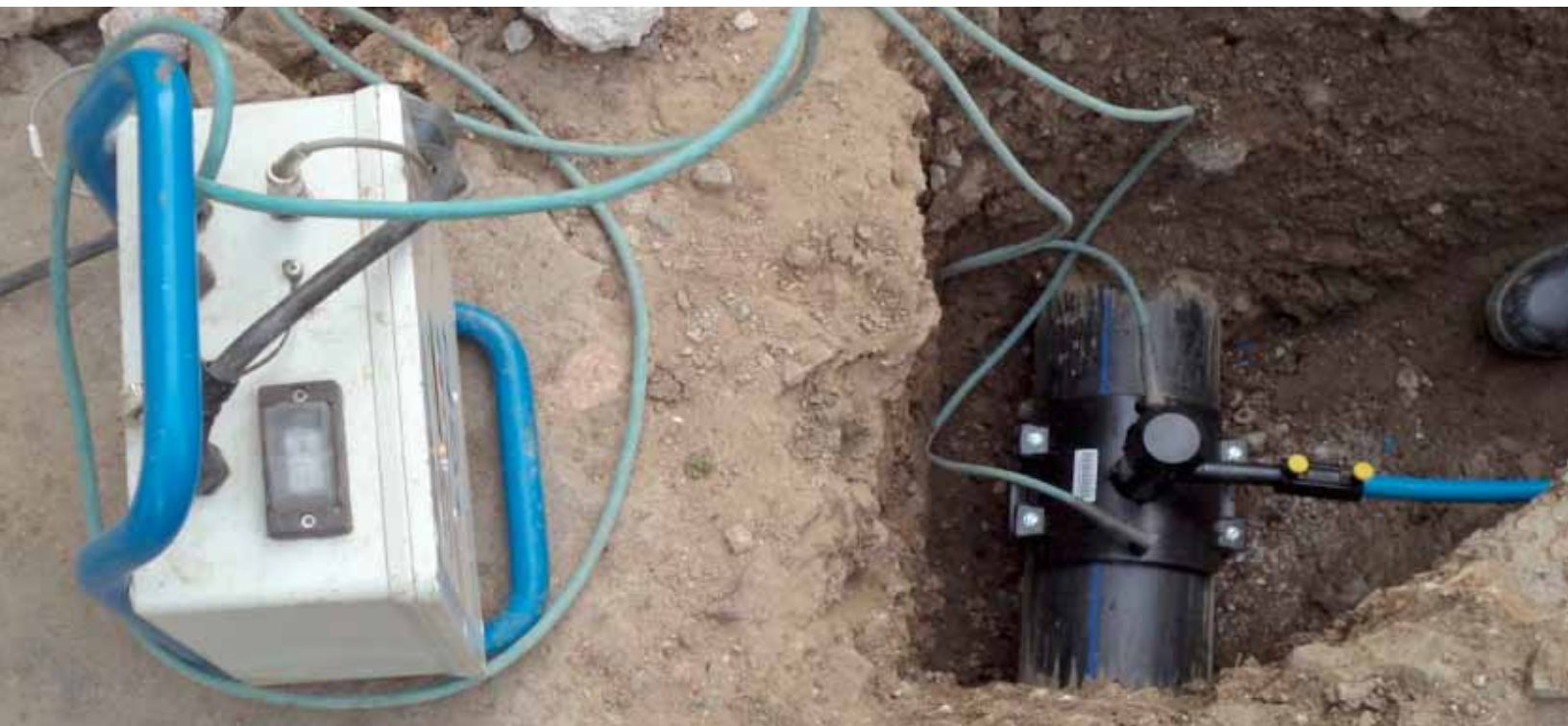
Electro fusion of saddle for house service connection (to ensure watertight joint).
